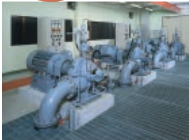
High-efficiency pump flow control
